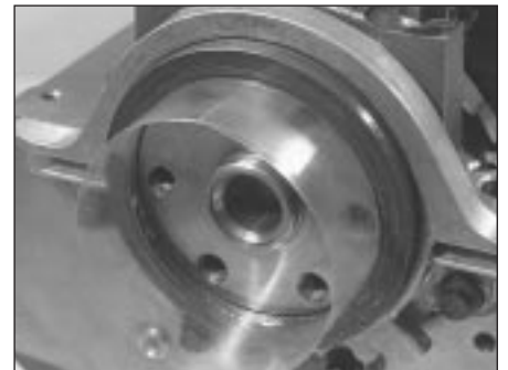
15.18 Using guide made from thin sheet of plastic to slide oil seal lips over crankshaft shoulder
