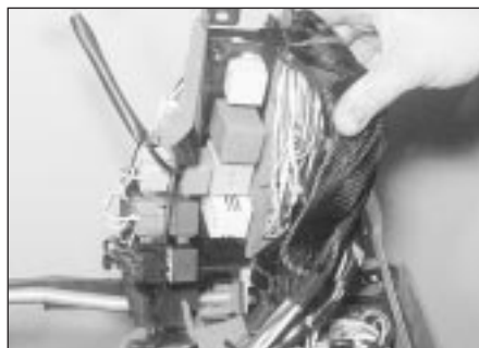
3.14c Main relay box located behind fusebox at rear of facia - models from 1993 (viewed with facia removed and inverted)
