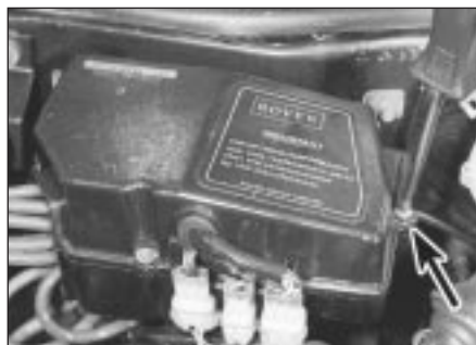
10.26 Undo the three screws and lift off the control box upper cover
