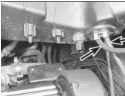
12.2 Thermac switch vacuum hoses (arrowed)
