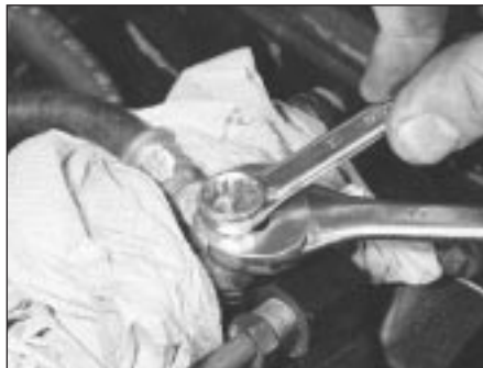
5.4 Releasing the fuel system pressure at the bleed screw on the banjo union
