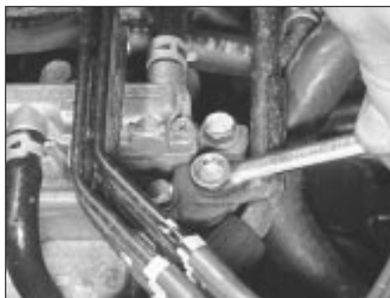
12.30 Undo the bolts securing the vacuum pipe and crankcase ventilation pipe support brackets
